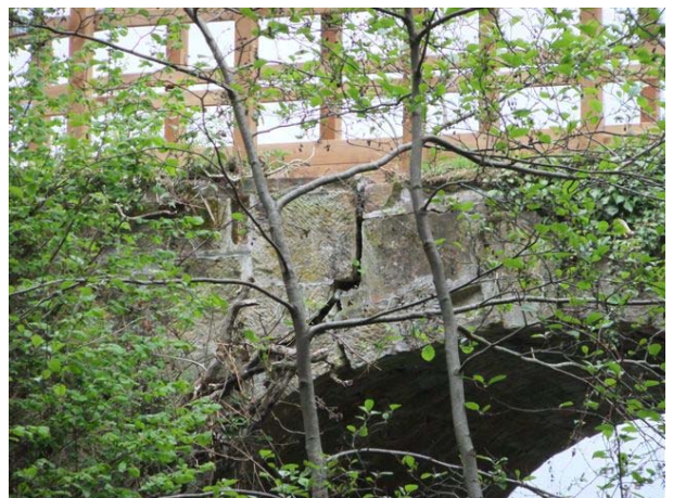
The picture shows the new structure at the top of the bridge, and the cracks that remain underneath
